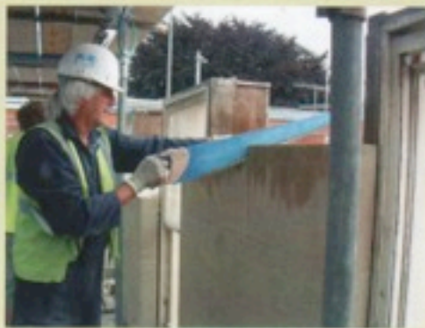
Existing mortar is cut to release stone without causing damage to face edges
