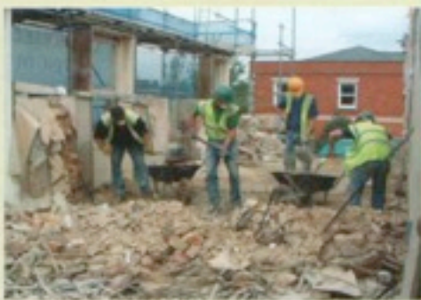
Reclaimed materials: brick, joists, floorboards, precious metals (copper, lead), other metals, internal doors, door hardware, woodwork, general fittings
